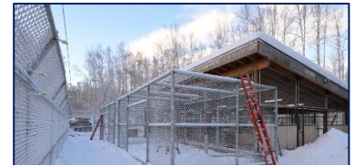
Figure 4. Modernization of the Summer Bear facility at UAF Large Animal Isolation Facility., winter 2025.
